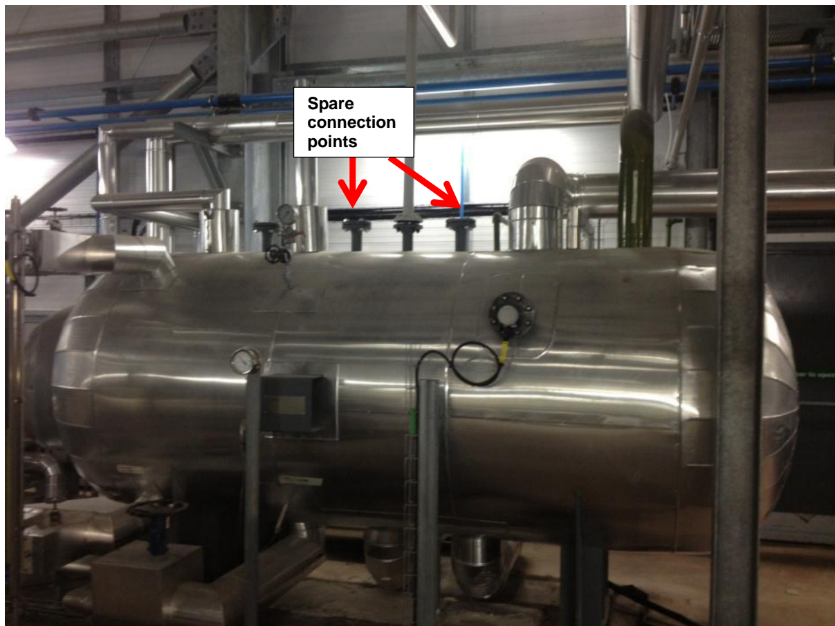
Figure 4-2: EfW condensate return tank with available connection points at top
